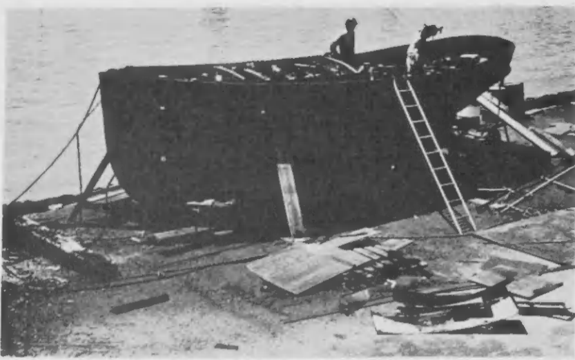
HAMMERS AND torches are being used on a stripped-down worklady of the harbor, known affectionately as Mooring Launch Number 2. She's getting a new gunwale and deck housing, and other needed repairs next to other projects at the drydock.
